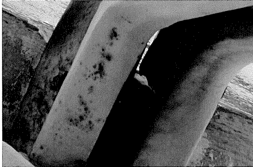
Photo Four: Extensive corrosion of rail section (between members). Surface corrosion and loose rust evident.
