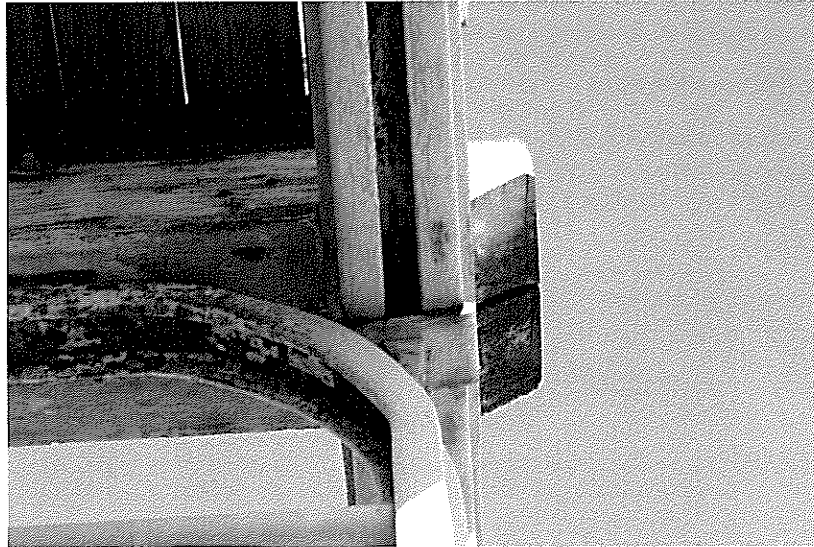
Photo Three: Timber corbel with split along bolt line.
