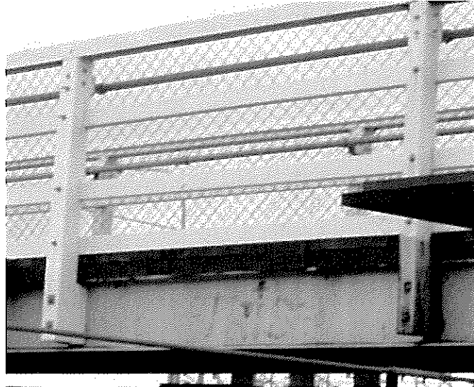
Photo Eight: Comparison of old and new balustrade supports
