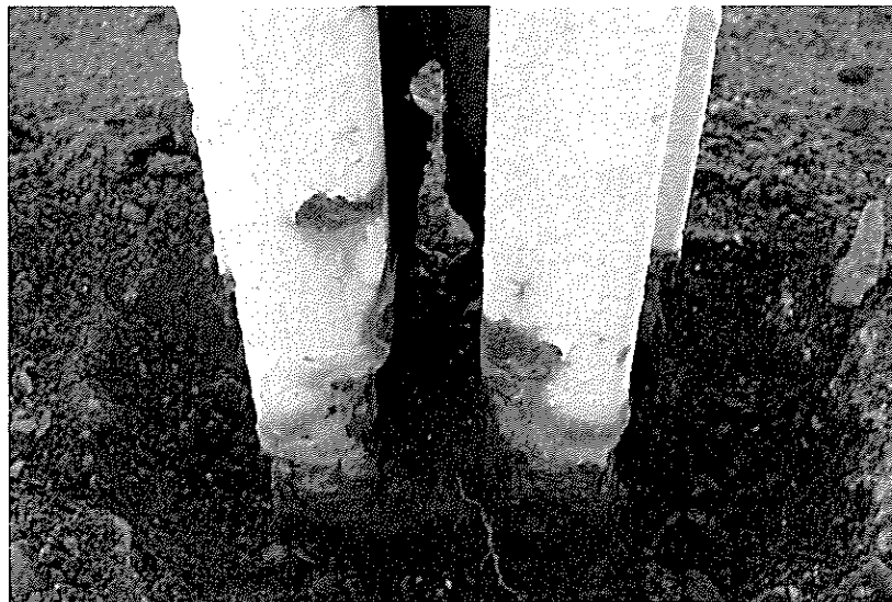
Photo Five: Extensive corrosion of rail and loss of section at base.
