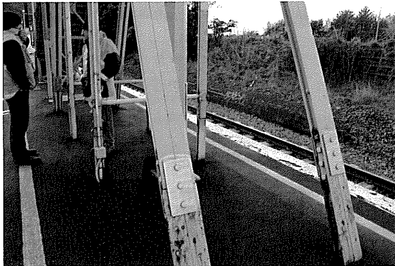
Photo Eleven: East side pier. Extensive corrosion to the pier leg connecting bolts and the circular hollow section prop between rail-iron legs. Note plates added recently at joint.
