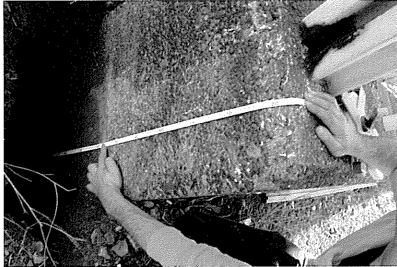
Photo Ten: Bottom of concrete pad foundation adjacent to the west boundary fence is 600mm below ground level, founded on solid ground.
