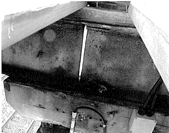
Photo Nine: Corrosion to the tops of the top flange of the I-beams under the timber packers supporting the deck.
