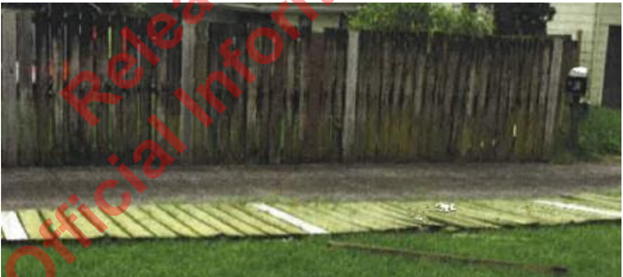
Above: Repairs to this fence line would exceed more than 50% of the replacement cost.
