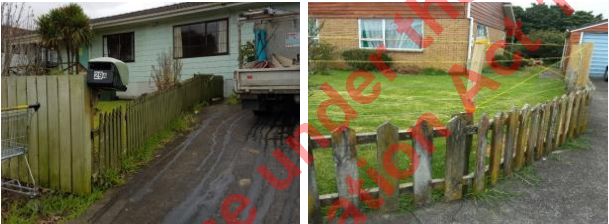
Above: Both fence lines are less than 900mm in height and should be replaced.
