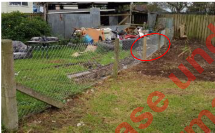
Above: Minor repairs have been carried out on the mesh fence. A new post has been installed along with a small section of new mesh.
