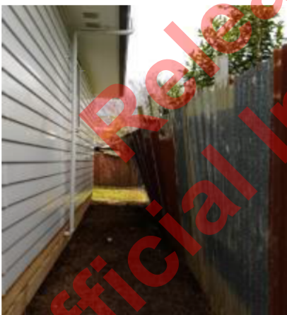
Above: Corrugated fences are not acceptable and shall be replaced with timber fences.
