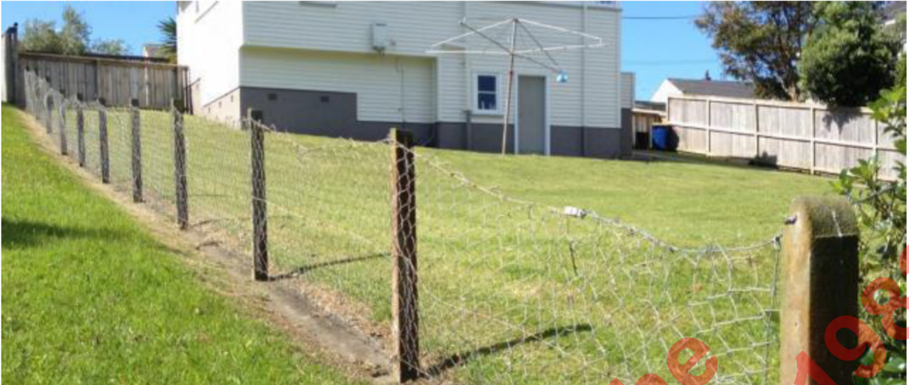
Above: Minor repairs can be carried out to bring this fence up to the required standard. The strainer wires require tensioning
