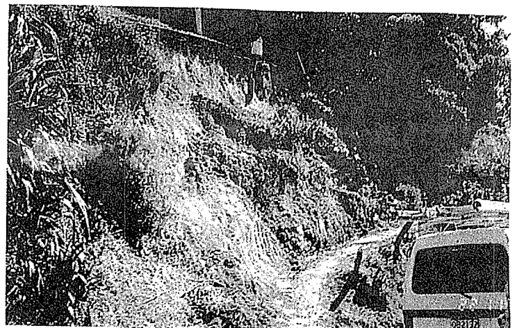
45 Kainui Road - Slip on legal road extending on to private property.
