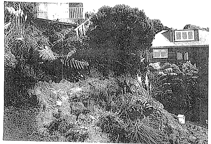
6A Kilsyth Street - Slip on private property, private pathway and house foundation undermined.
