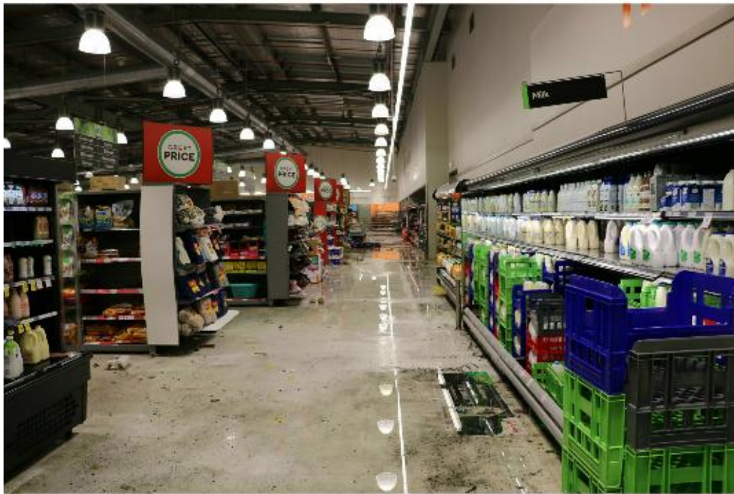
Photo 17: The rear of the supermarket looking towards the dairy and meat departments.
