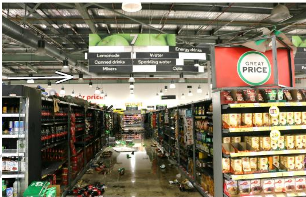
Photo 21: Aisle number 7. The fire travel from aisle number 6 into aisle number 7 through the back of the shelf is shown by the white arrow.
