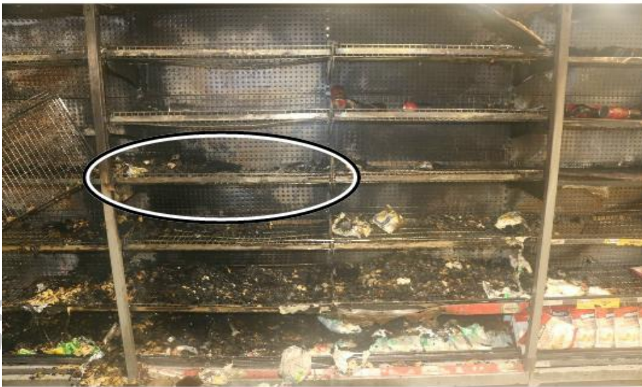
Photo 23: The section of the shelving units where the fire originated from. The shelf that the fire started on is shown by the white circle.
