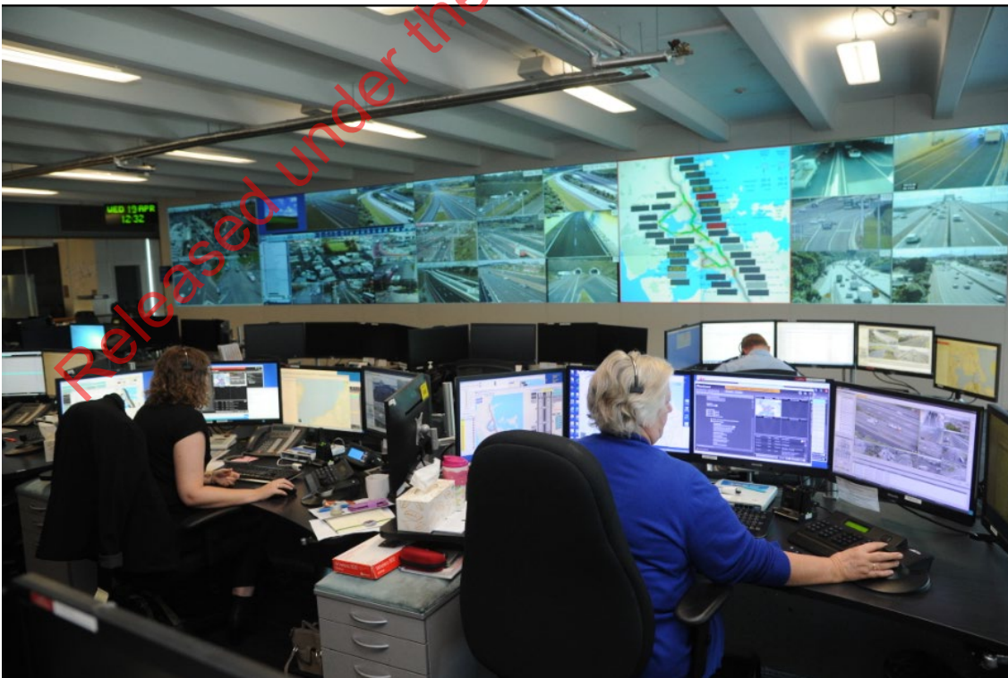
Figure 1. TOC Operations Room
