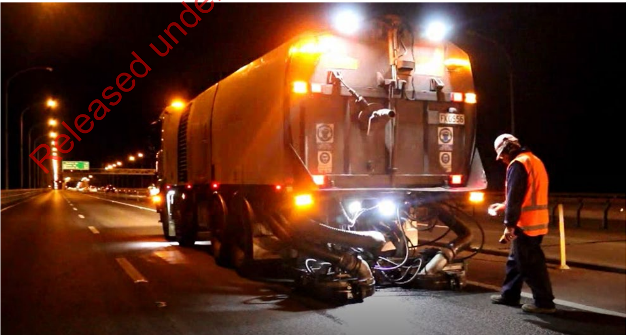
Figure 24. Captive water blaster is used to remove material from the voids in the OGPA.
