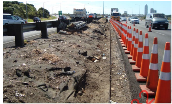
Figure 27. Damaged median barrier delineated by traffic cones prior to opening adjacent lane under reduced speed limit.
