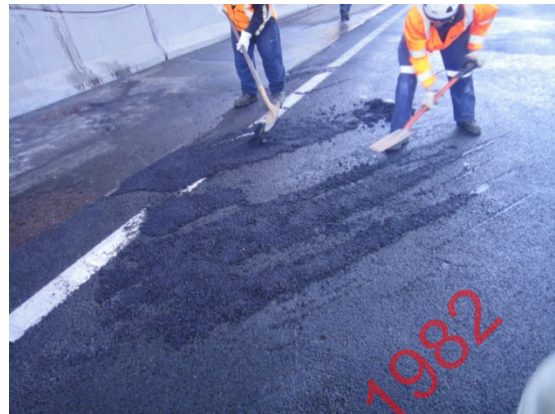
Figure 30. Gouges and deep scrape marks must be filled prior to re-opening of road.
