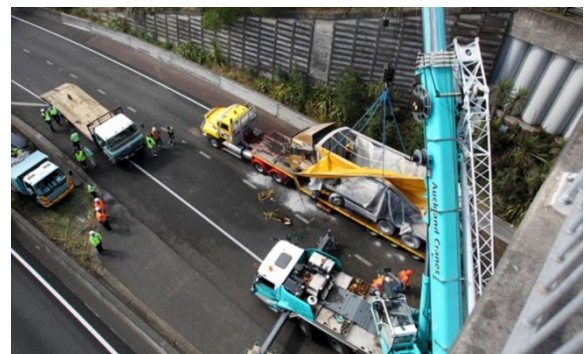
Figure 20. Deployment of cranes on or near structures must be approved and monitored by the bridge engineer.
