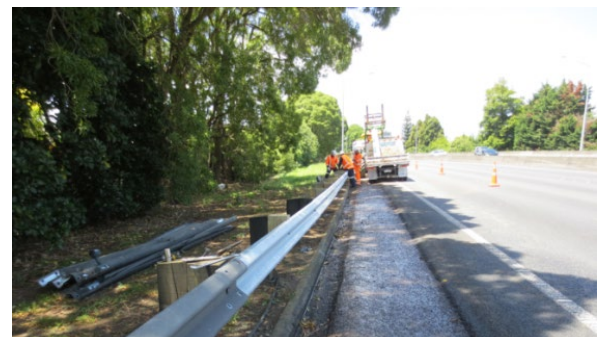
Figure 29. Permanent repairs can sometimes be completed on site with minimal disruption to traffic operations.
