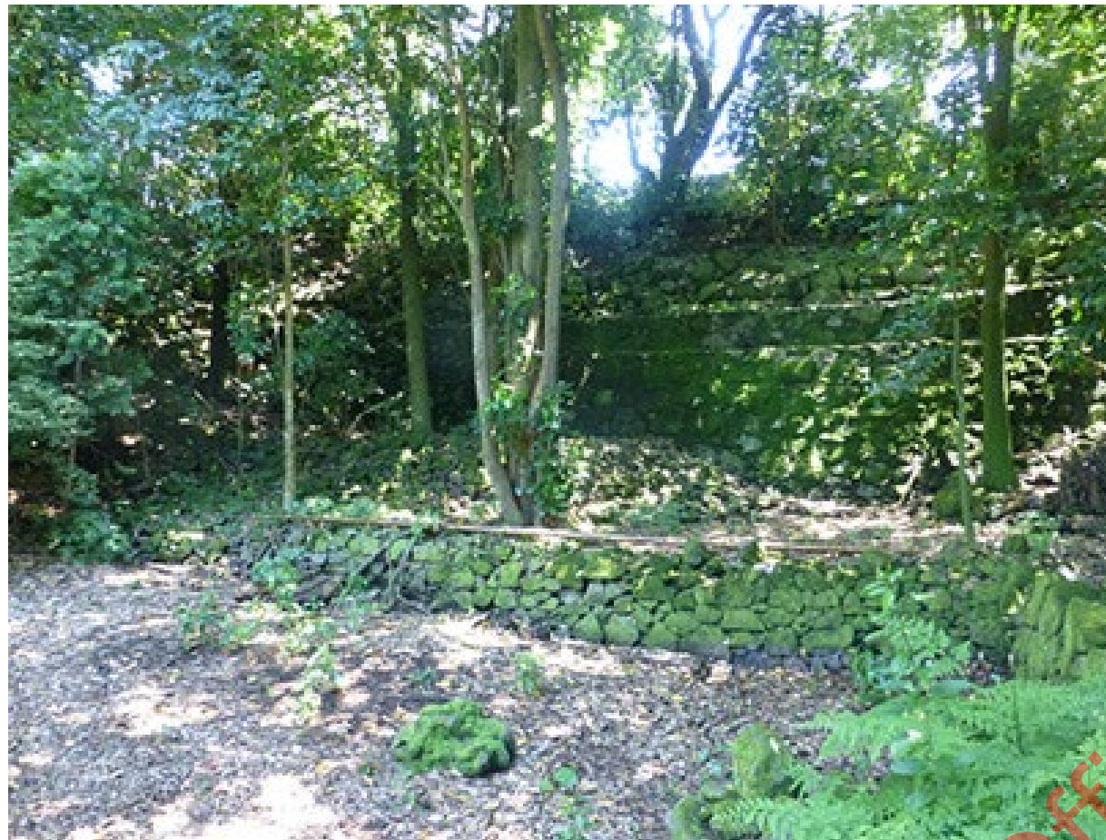
Early retaining walls in north east corner of Glenfell Place Rock forest area
