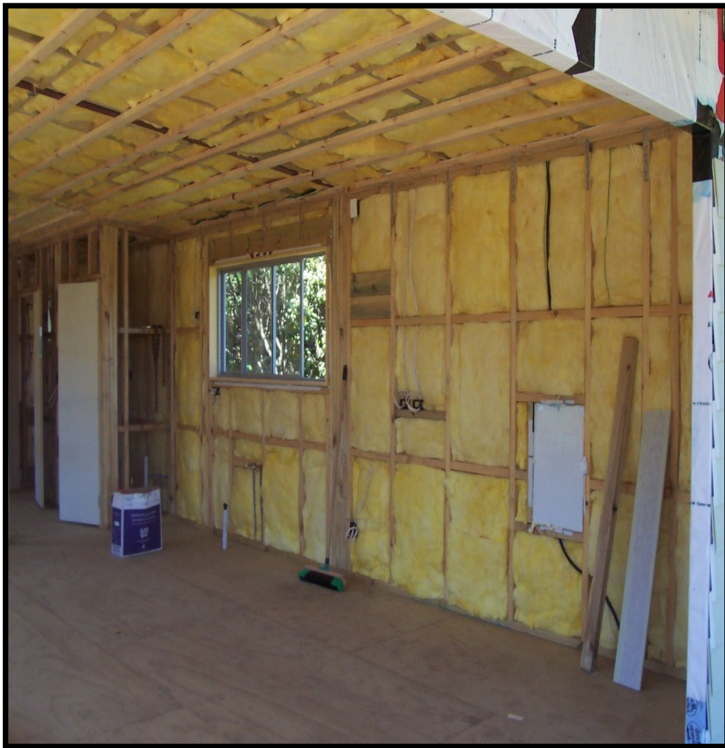
Figure above: preline build inspection unachievable because building is not weathertight.
