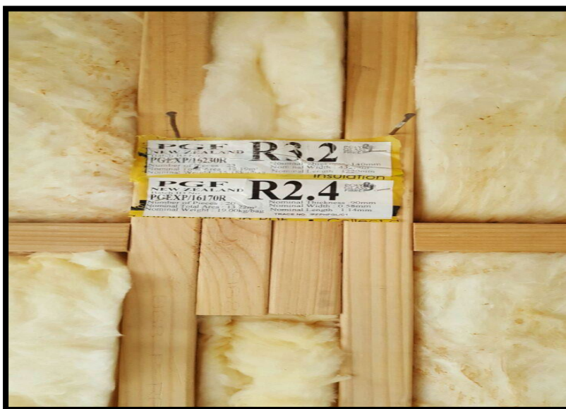
Figure above: sample of insulation tags
