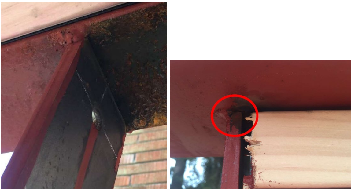
Figure 163. Look out for welds on one side only. All welds should be both sides of fillet.
