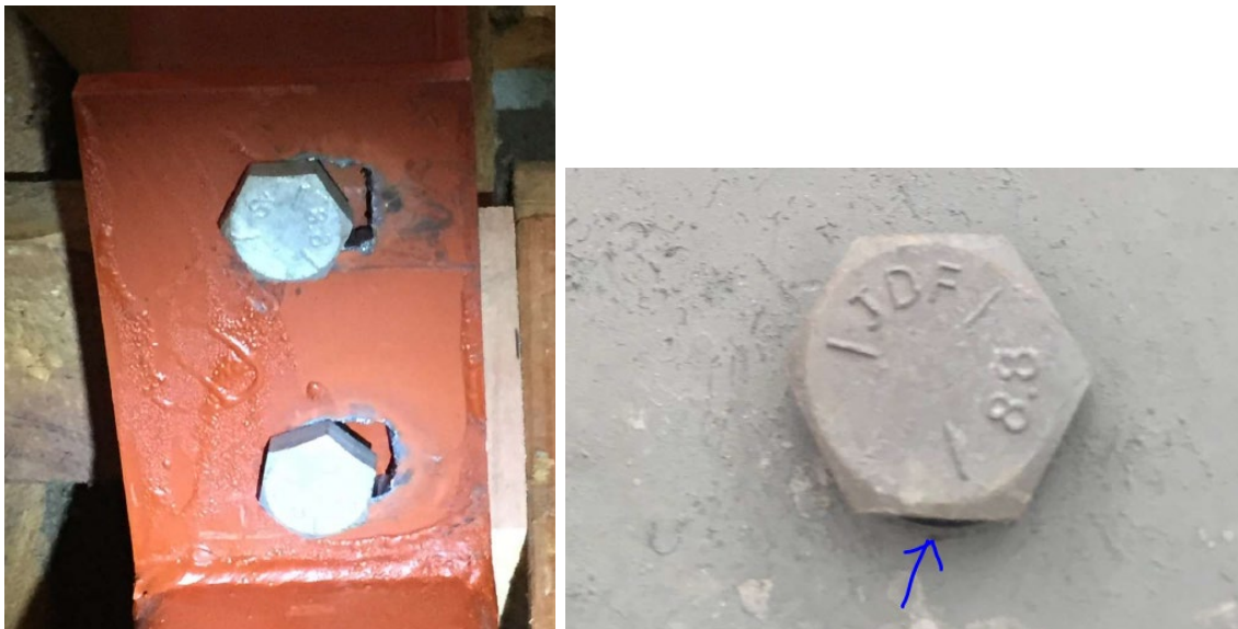
Figure 154. Where bolt holes are oversized, a heavy washer may be used but this should be specified by an engineer. Note: Check the 8.8 bolt on the right is the correct bolt to use by looking at engineers' specifications.
