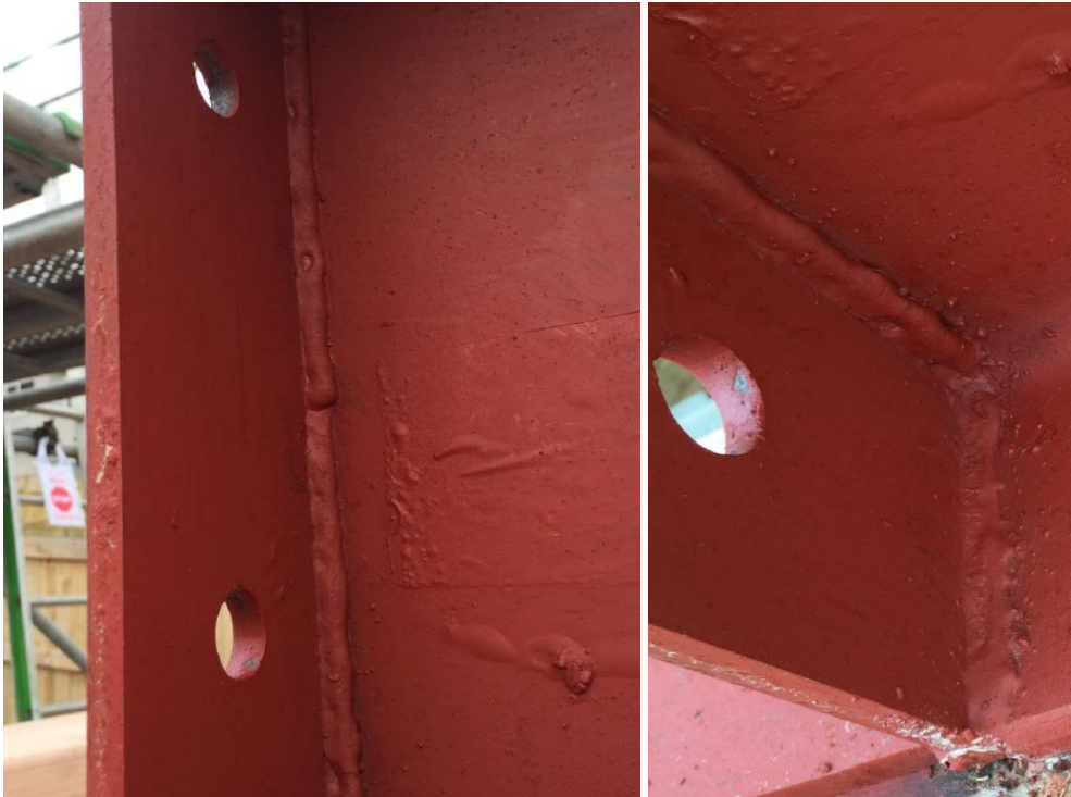
Figure 164. Flux build up not removed masks the true weld size. Once removed, these welds were shown to be too small.
