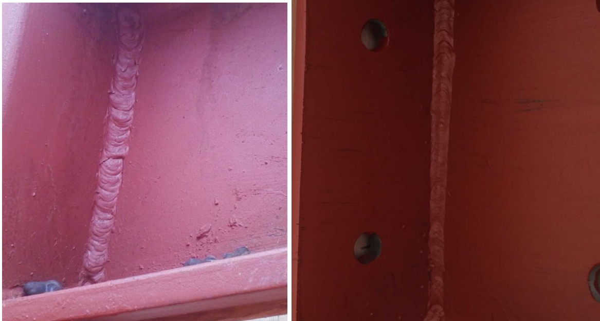
Figure 158. Good clean even welding is easy to identify visually. Note: this visual inspection does not take the place of the ITP.
