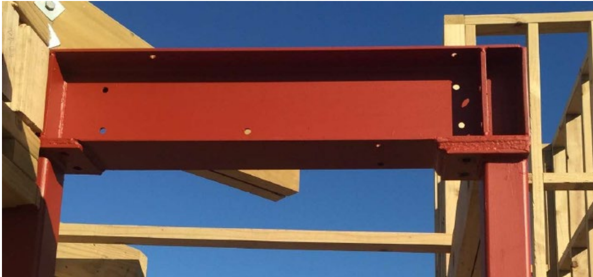
Figure 155. When a bolted joint is specified and welding is used instead, this must be approved by the structural engineer and registered as a variation on the consent.
