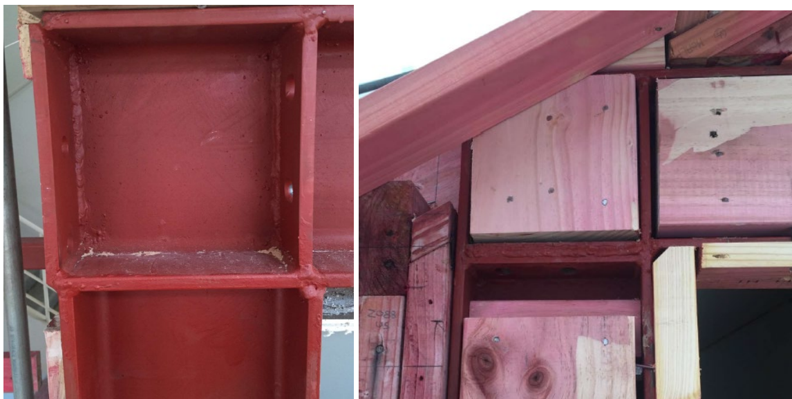
Figure 165. Misalignments need to be referred to an engineer to inspect and approve or provide remedial instructions. Note the misalignment was rectified above by welding extra steel plate to strengthen the joint.
