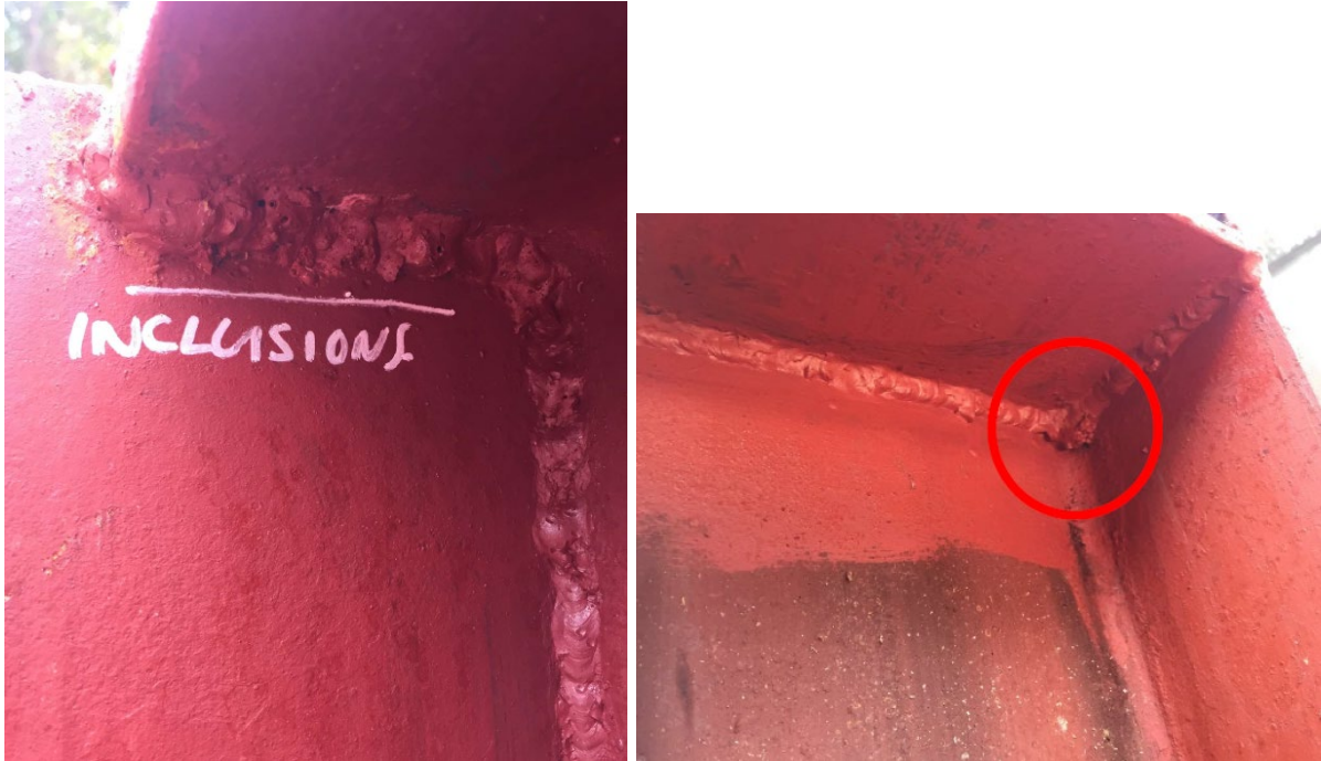
Figure 162. Inclusions can build a weld up to look thick enough but in reality it would have the effect of having no or little weld in place.
