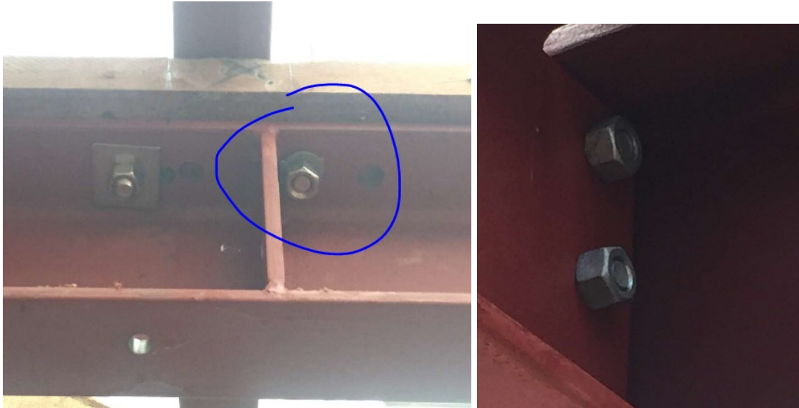
Figure 153. Inspectors should see one full thread past the nut and washers installed.
