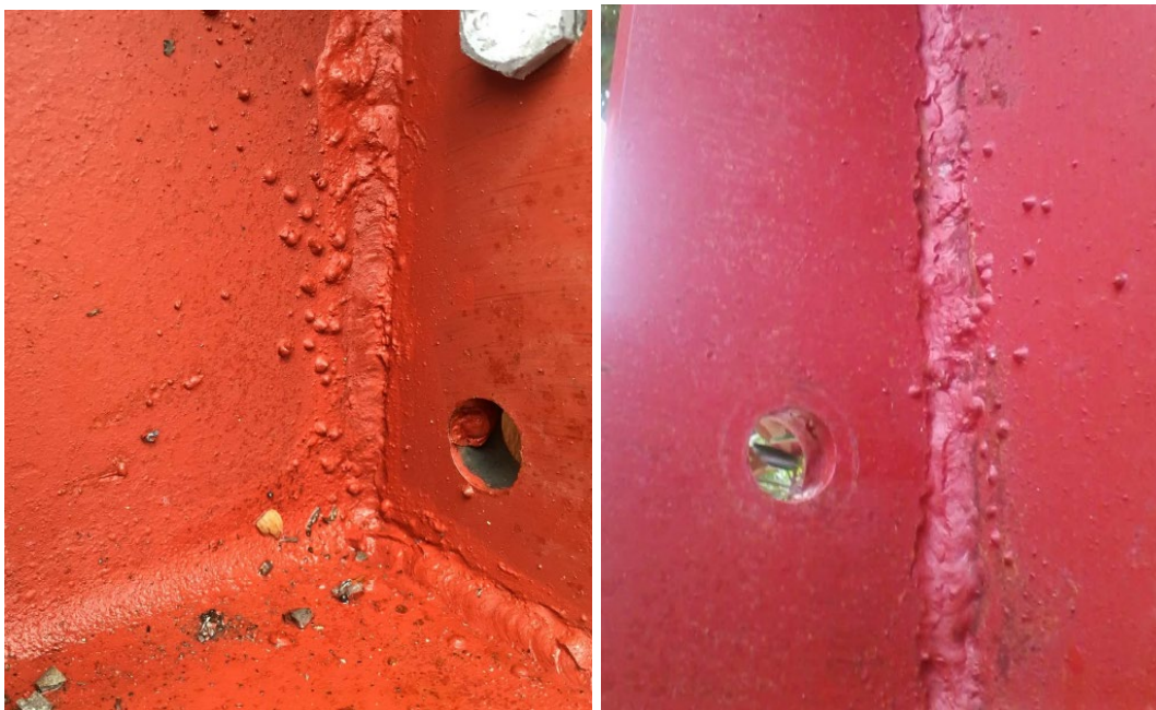
Figure 161. Sometimes, spatter leads your eye to other issues. In these cases, the welds are “undercut” or lacking fill. There is insufficient weld to provide structural adequacy.
