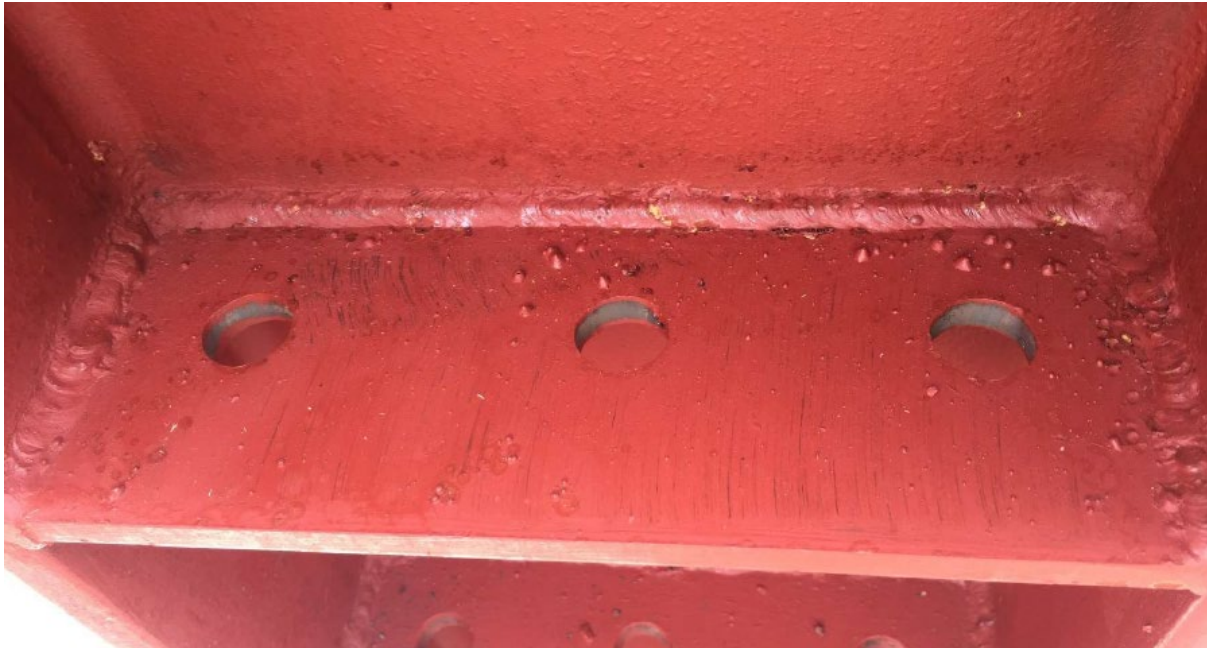
Figure 160. Shows heavy spatter from arc blow resulting in a small weld.
