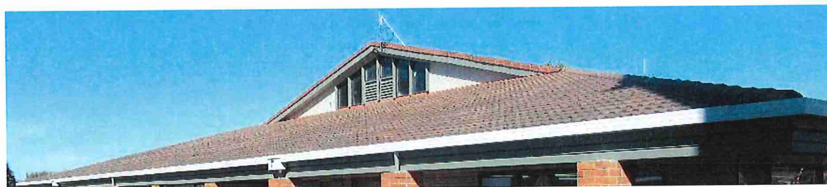
Image showing the tiled roof with hips in the corners and a part gable above the central core wall.
