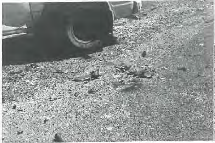
Fig 7. Gouging to westbound lane visible in centre of view and highlighted by orange paint.
