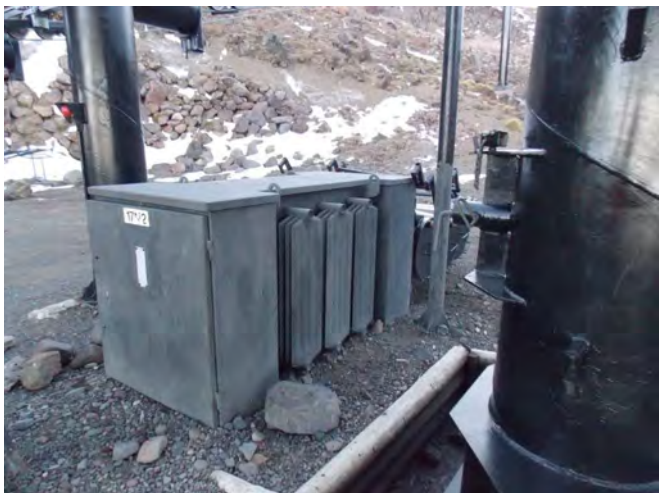
Existing T17N02-300KVA Ground Mount
