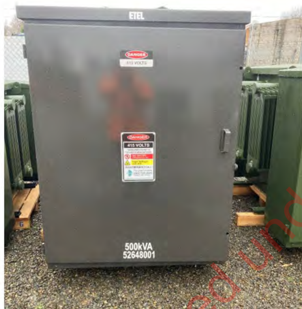
New 500KVA Ground Mount
