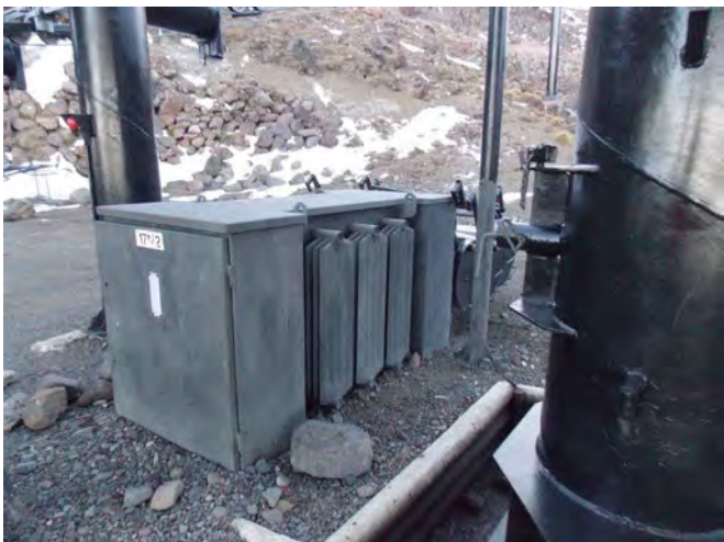
Existing T17N02-300KVA Ground Mount
