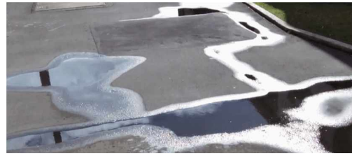
Figure 18: Puddles show uneven surface
