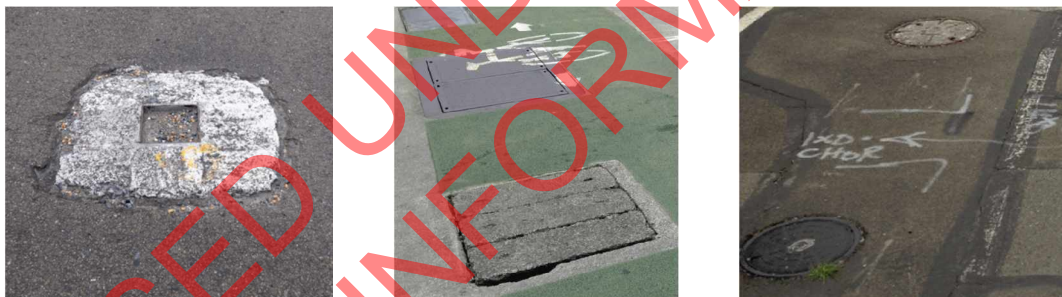
Figure 21: Path surface hazards
