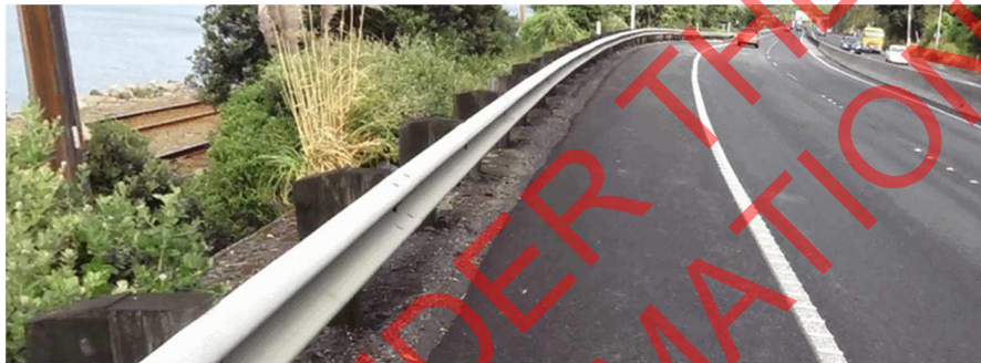
Figure 57: New path will have similar constriction issues here as per Section 3 Option 1 Figure 58 shows more of the same safety and user issues at CH 4,100 as per 3.3.3.
