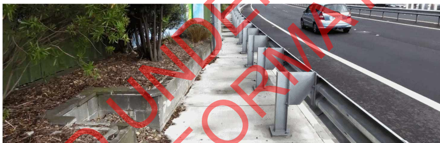
Figure 62: Limited space between guardrail and built structure
