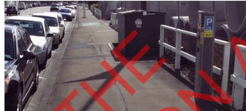
Figure 10: Utility transformer and parking meter
