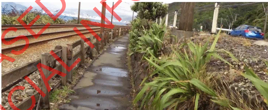
Figure 53: : Fence, poles, retaining wall, trees, deflecting wire rope and road at head height
