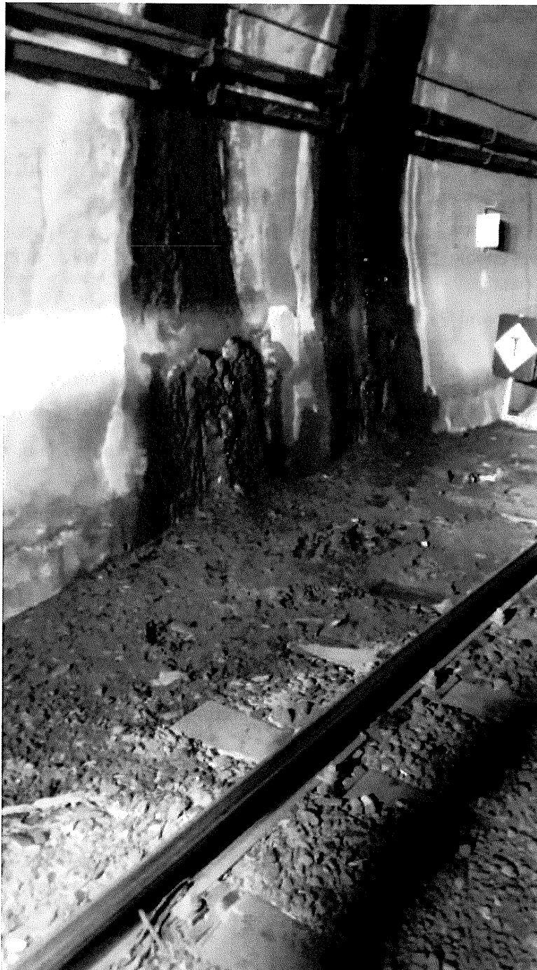
Figure 23 – Water ingress in Rimutaka Tunnel leading to deterioration in track and formation.
