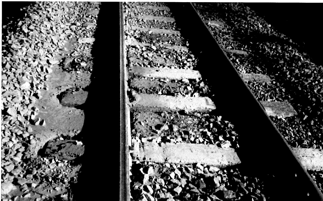
Figure 16 – A mudspot – failed formation under track - leading to loss of track geometry and the need for repeated intervention (continual repairs) in the absence of proper renewal.
