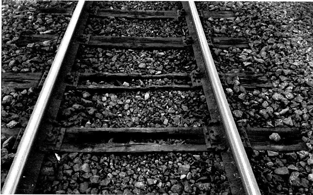
Figure 15 - Deteriorated Treated Pinus Radiata (TPR) sleepers. These are endemic on the Wairarapa Line, with the sleepers replaced during significant volumes of renewals nearly 40 years ago now having run through their life cycle
