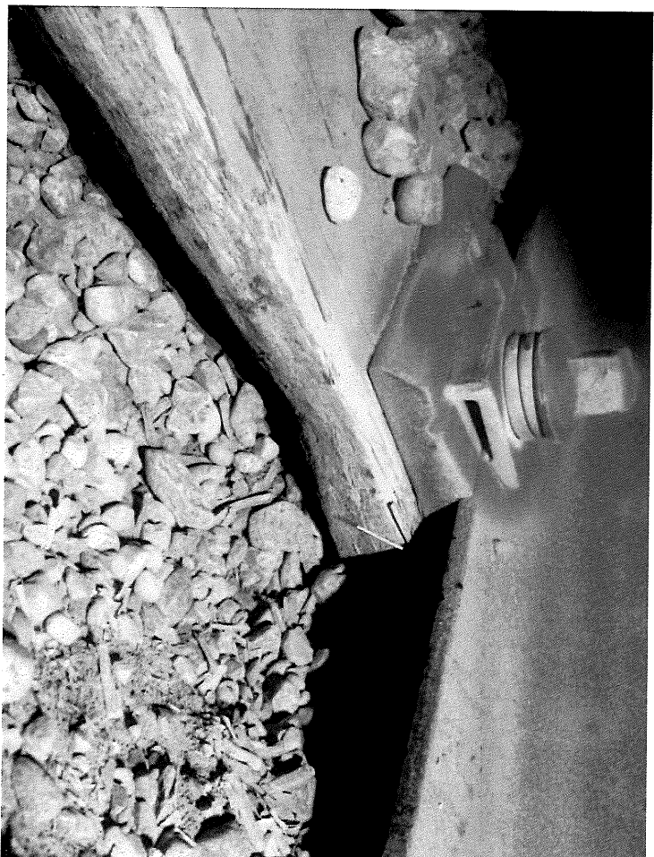
Figure 28 – End of Life and Poor Condition Track Tunnel Photos (Tunnel 2 WL)
